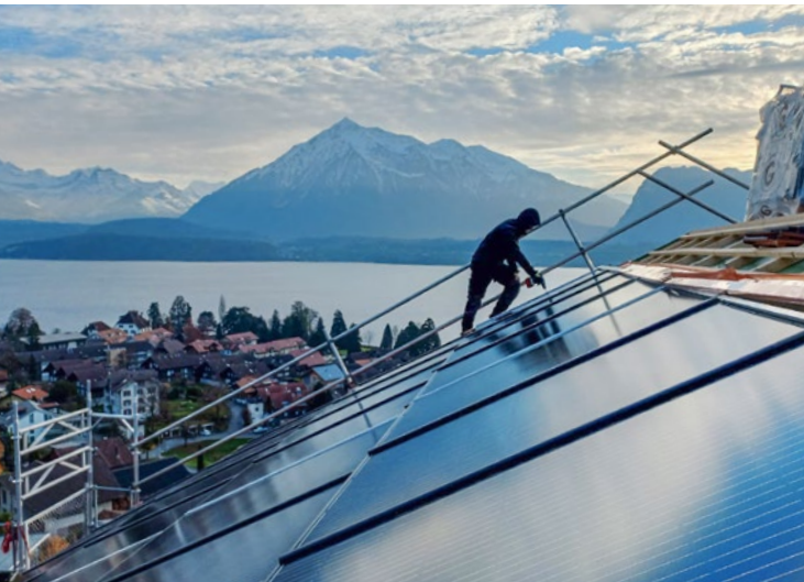
Installation Photovoltaik Oberhofen
